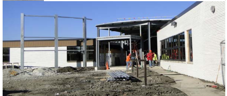
Fenton's new main entrance in late October. Steel work started and plans for pavers implemented.
