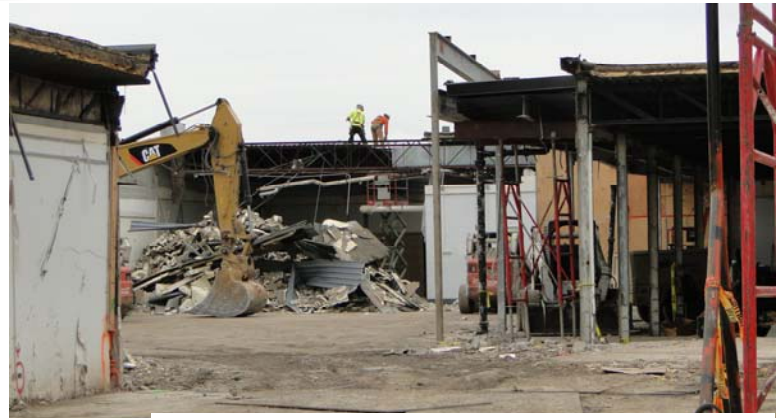
Demolition to make way for the new main entrance began in the summer and continued through October.
